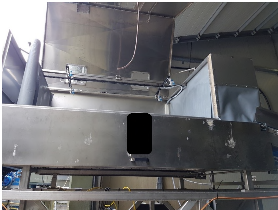
Picture 1: fixed disinfection enclosure (open) in the disinfection cell
