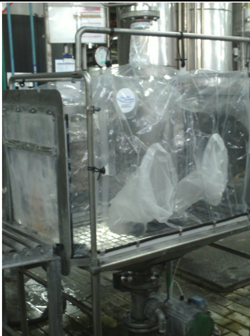
Figure 4 Enclosed Sodium Hydroxide charging booth
