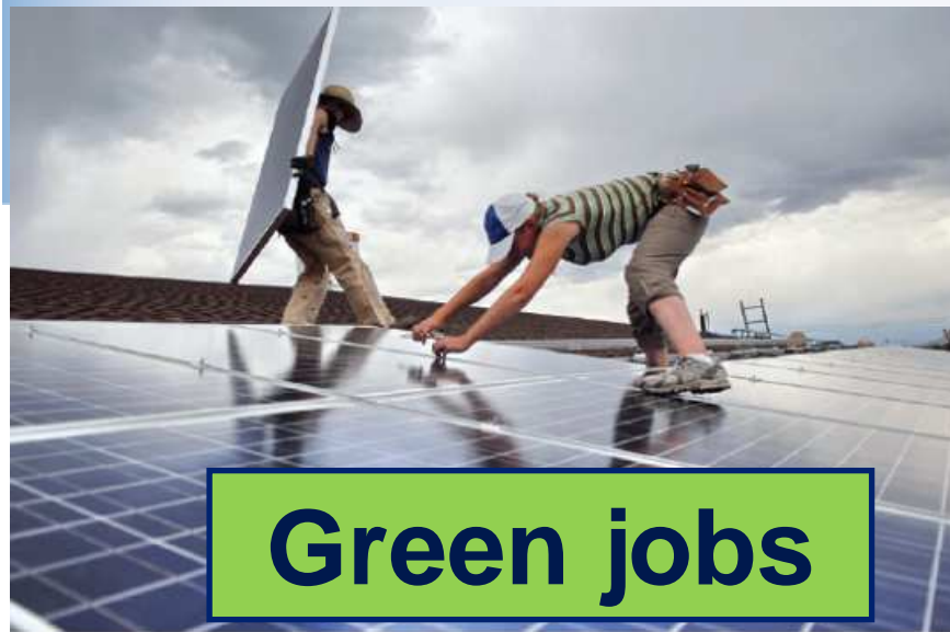
Louisville-based Bella Energy worked with EMC Engineers on this photovoltaic installation for the Antonito School District in the San Luis Valley of Colorado.
