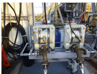
Pumps with flush lines
